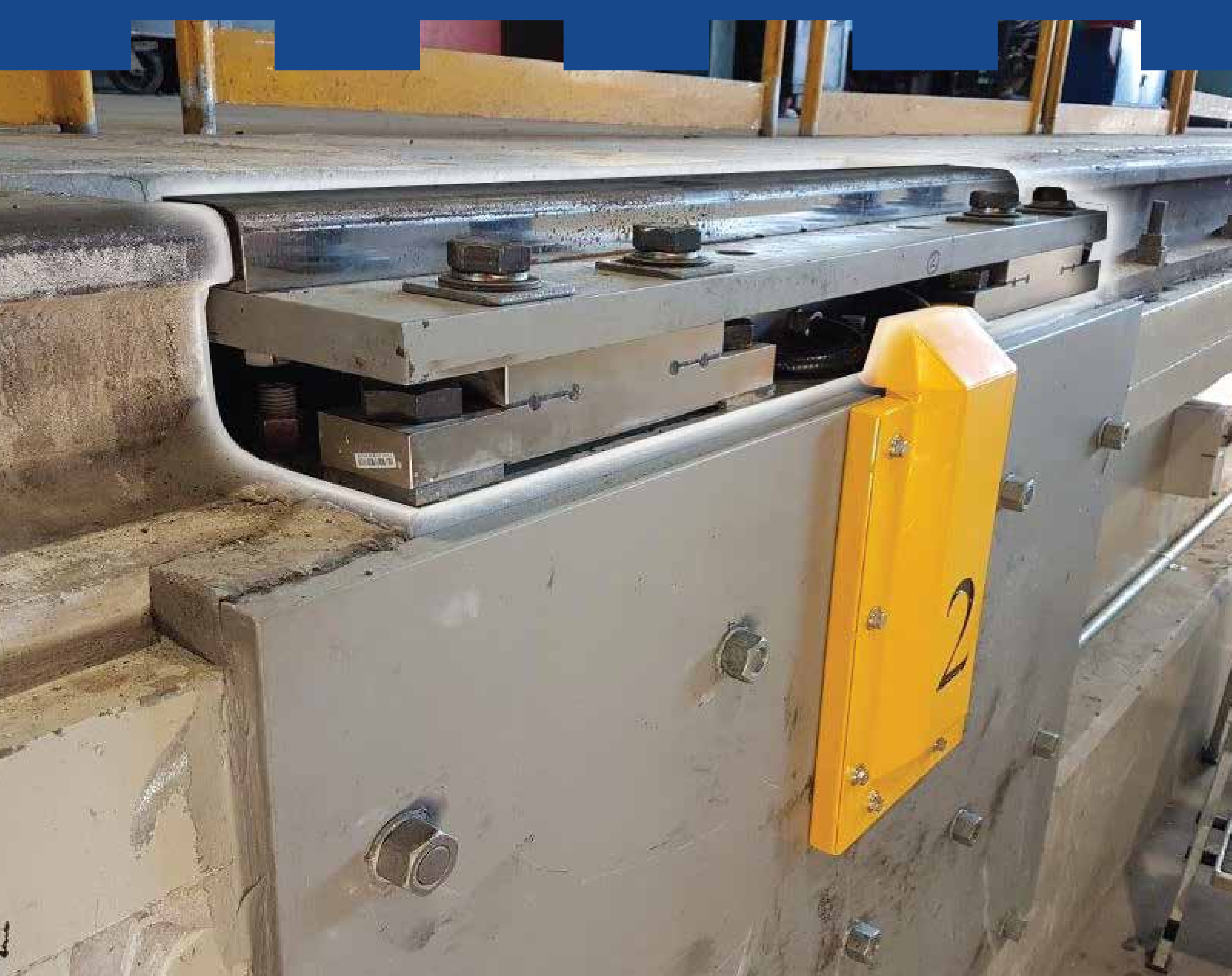
TRAKMATE installed within a Rail Workshop
